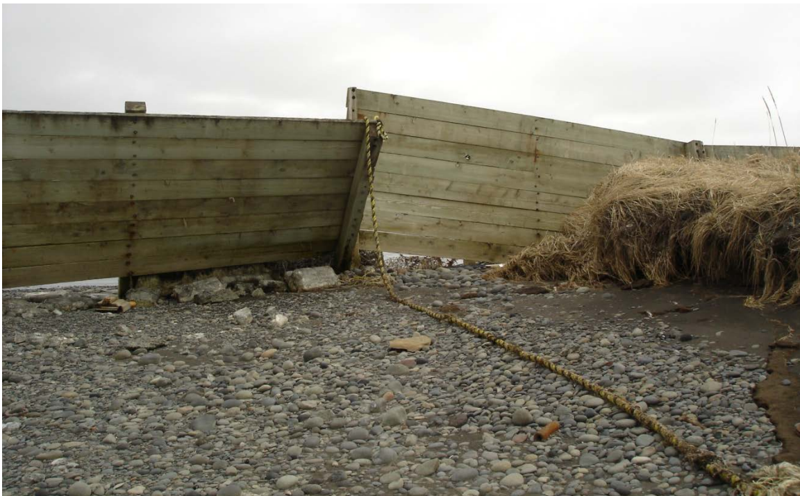
Figure 18. Damage to Wooden Seawall
